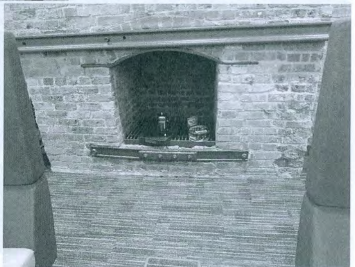
The corresponding smaller GER furnace on the south side. The fire bars appear a modern replica.
