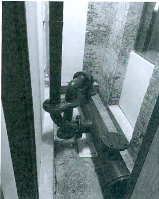
Ground floor view of the large diameter water pipes supplying the overhead water tank. [Photo PCC 9 11 2018]
